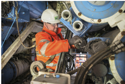
Top: Container stores on site guarantee the rapid replacement of wear parts.
